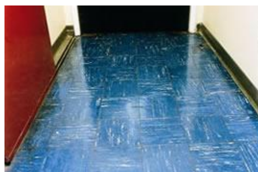
Asbestos containing floor tiles in a corridor
