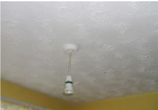
Asbestos textured coating
