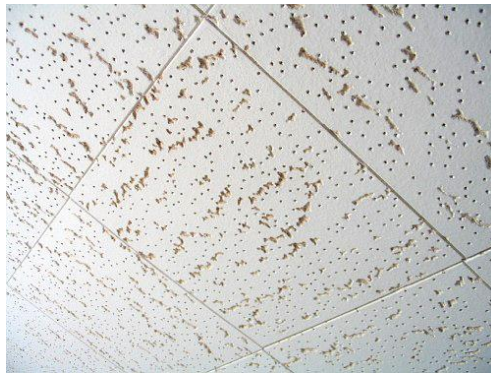
Asbestos containing ceiling tiles
